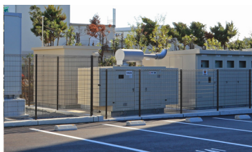
Emergency power generator
