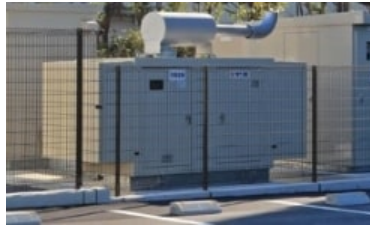
Emergency power generator
